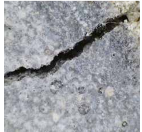
Concrete beam without AQUAFIX (0.5 mm crack)
